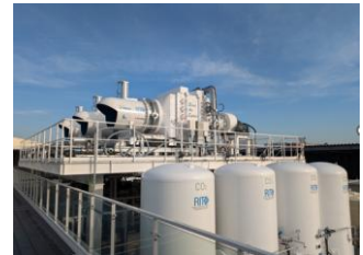
CO 2 Storage tank
